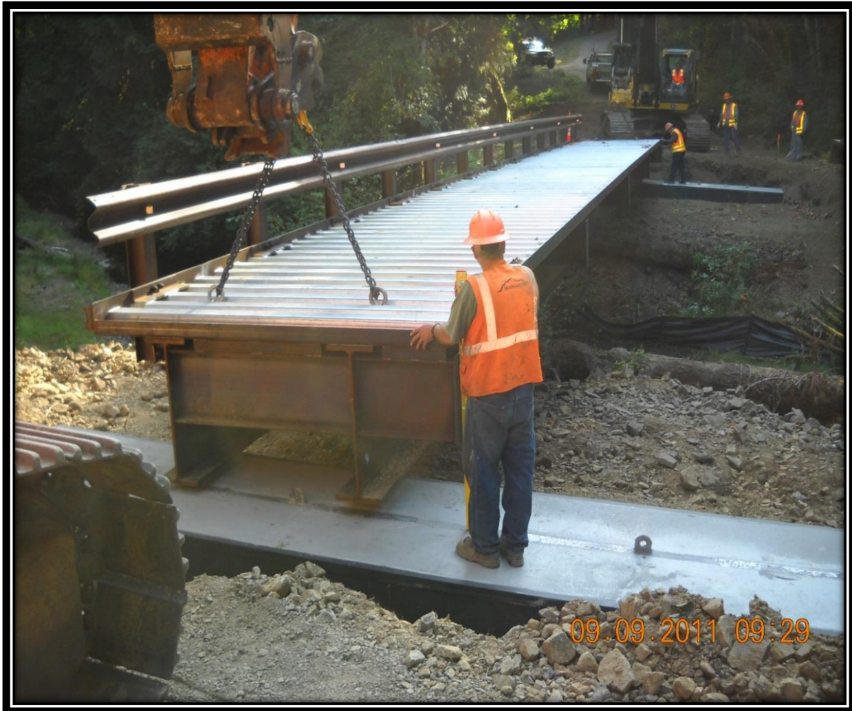
Cowlitz County Road Crew installing a modular steel emergency access bridge intended to provide alternate access during flooding that frequently closes Ostrander Road.
